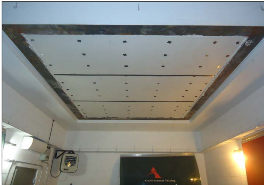
Source Room View of Test Specimen Installation
