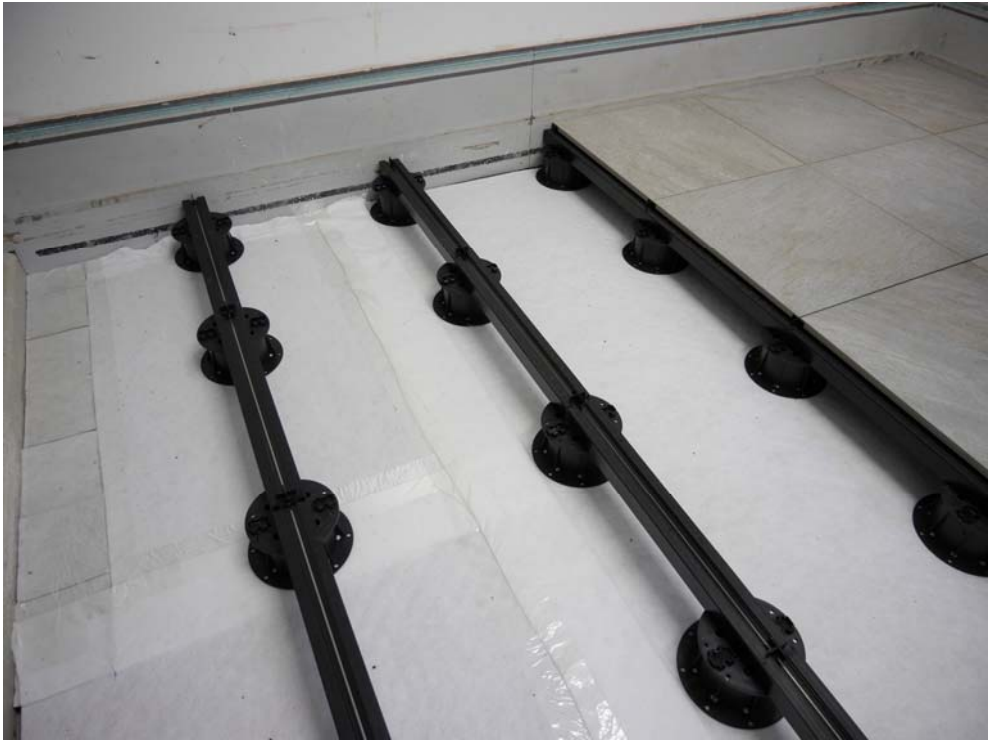
Figure B.3. Test setup during mounting: support profiles on pedestals and impact sound insulation layer.
