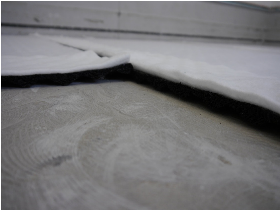
Figure B.1. Laying of the impact sound insulation layers Regupol® sound and drain 22 on the concrete ceiling slab.
